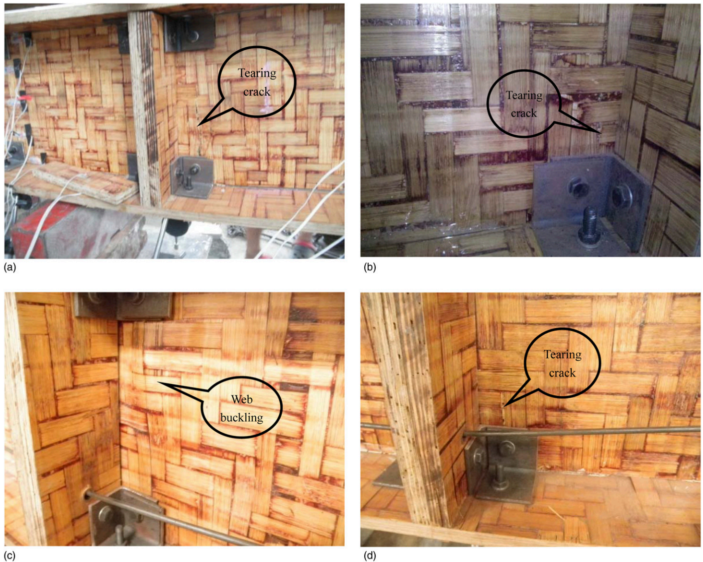
Fig. 6. Failure mode of four test beams: (a) Beam 1; (b) Beam 2; (c) Beam 3; (d) Beam 4 (images by Wenqing Wu)
